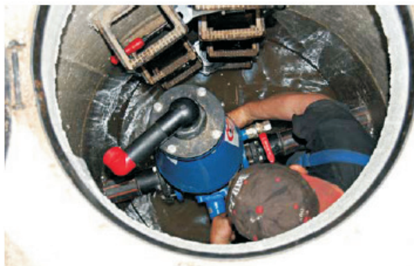
Fig. 1. Disassembly of the deaeration and aeration valve in a manhole \varnothing 1200 mm (conditions of life and health hazard: the practice is that the valve is disassembled after previous entering the manhole, and then it is taken to the workshop).
