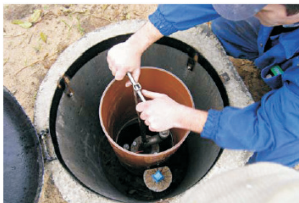
Fig. 2. Safe disassembly of the valve from the ground surface (the valve is replaced with a valve in working order, or a stopper is installed).
