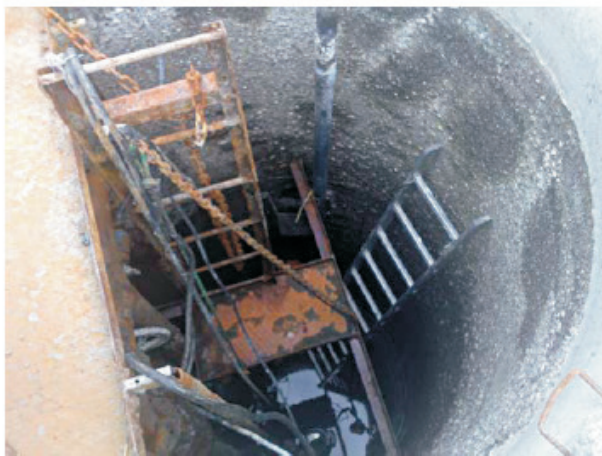
Fig. 3. A classical pumping station with a wet chamber and submersible pumps after several years of operation
