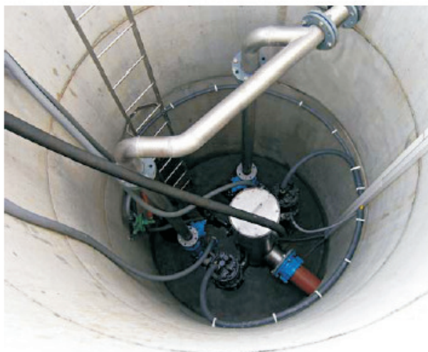
Fig. 4. Pumping station with a dry chamber and pumps in the dry mode after several years of operation
