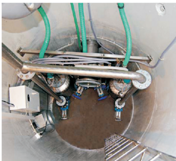
Fig. 5. A pneumatic sewage pumping station with working displacement tanks in the dry chamber
